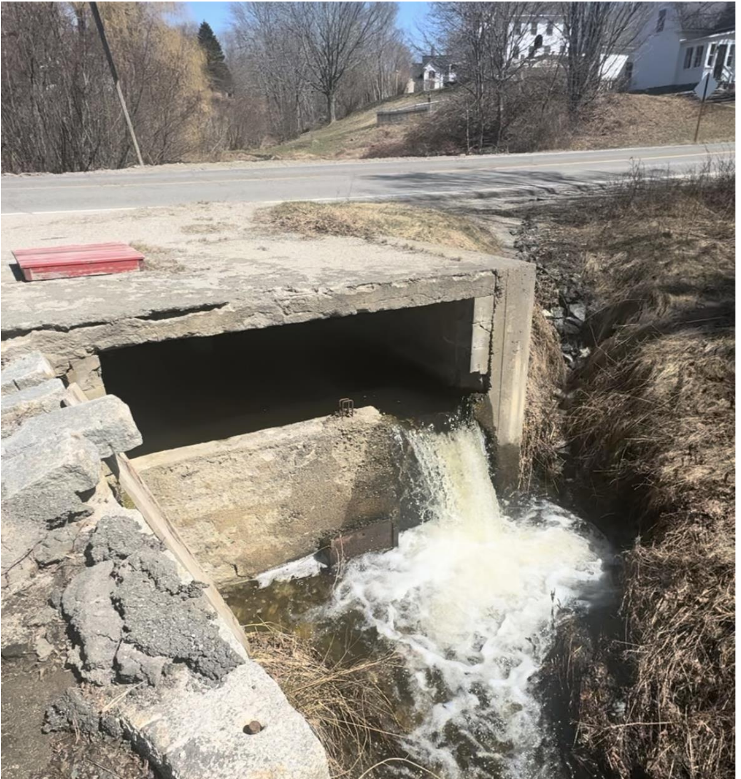
^Downstream side of the culvert showing the crumbling fire water cistern and heavy flows impounded causing pooling, standing West of State Highway Route 15, looking East. Photos taken April 5 th , following heavy rain events on March 23 rd and April 4 th .
