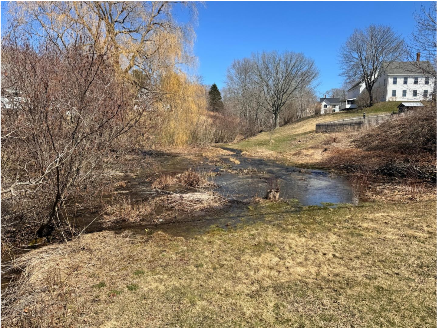
^ The upstream side of the culvert, standing on State Highway Route 15 looking East, flooded stream due to inadequate culvert size and flow.
