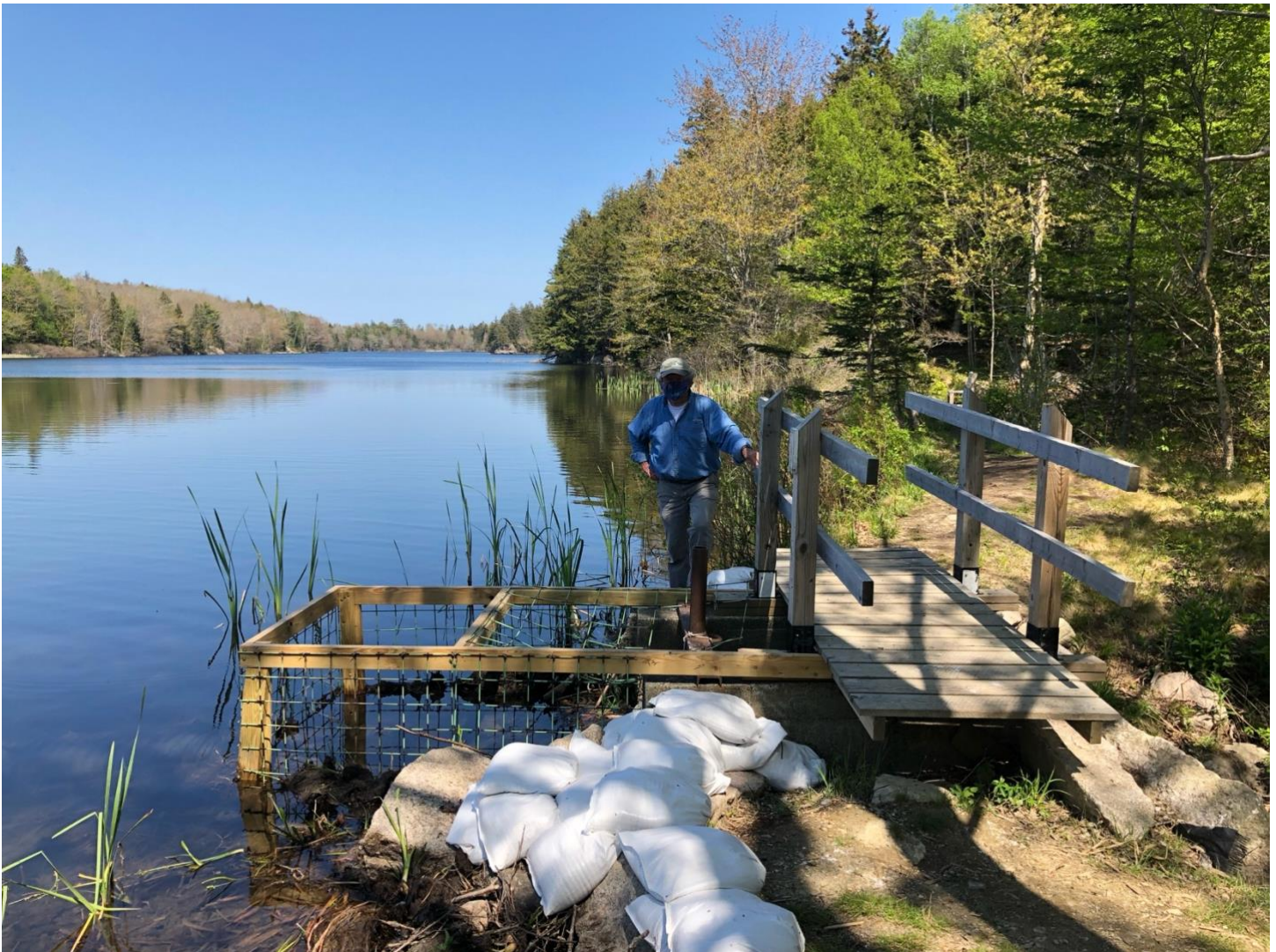
^Sandbagging areas on both sides of the spillway that showed evidence of overtopping. May 2020.
