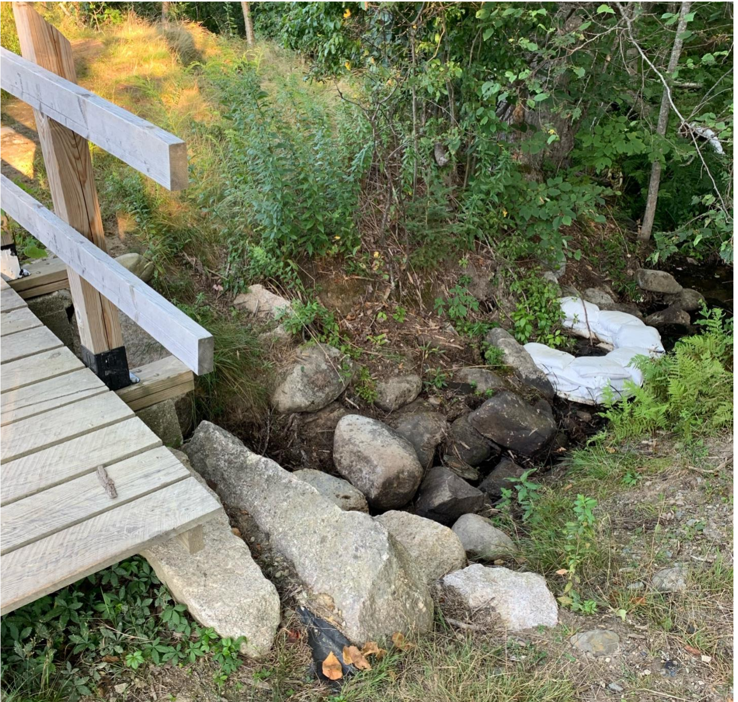
^Sandbagging around a boil in the outlet stream below the spillway. July 2021.
