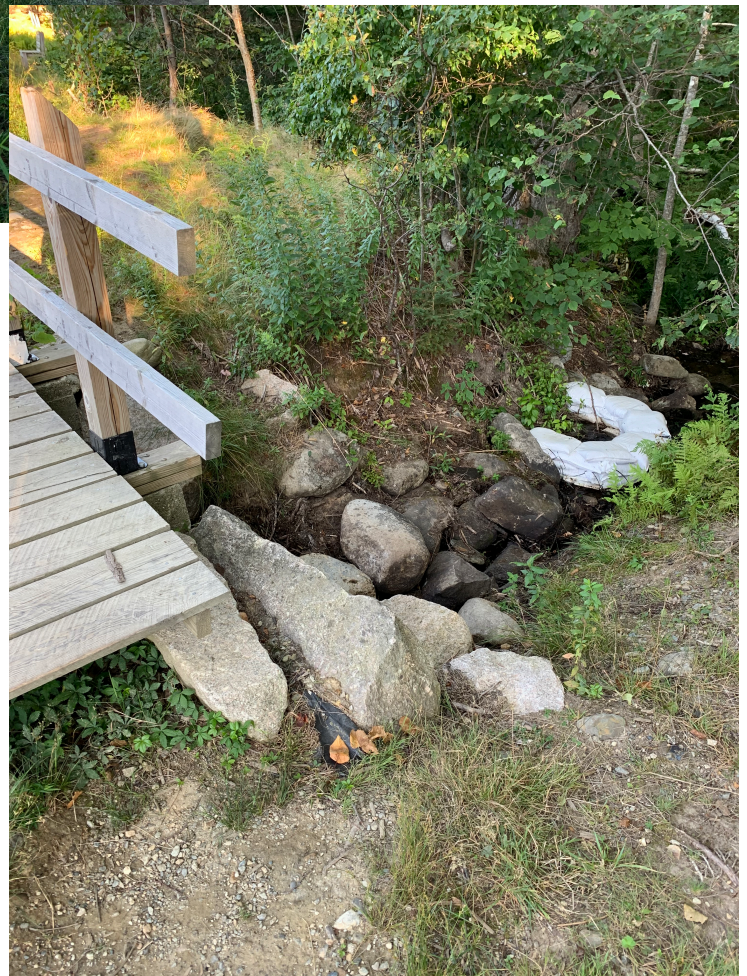
Looking at the outflow side of the spillway and to the sandbags around a "boil" downstream. Photo by Joe McLean >
