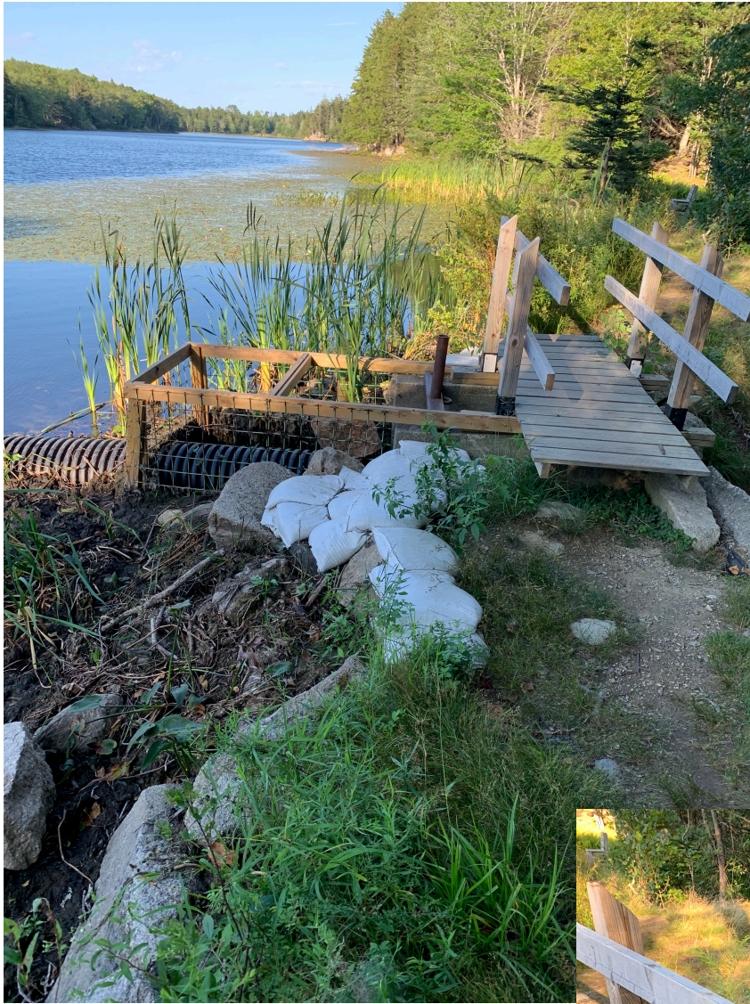
< On the dam crest facing NE. Current undersized spillway and walkway with beaver deceiver pipe and structure inflow. Sandbags have been placed around sites of previous over-topping. Photo by Joe McLean.
