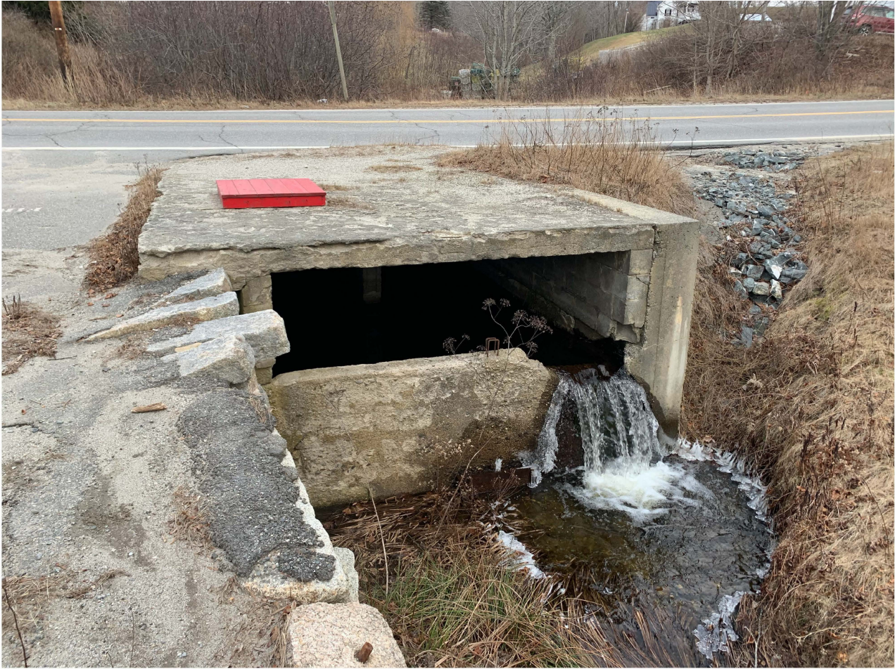
< SW side of Route 15 with the firewater cistern and access hatch. Photo by Joe McLean.
