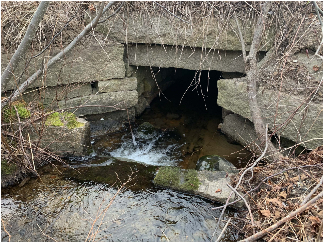
<NE side of the Route 15 culvert, currently undersized for the stream. Photo by Joe McLean.
